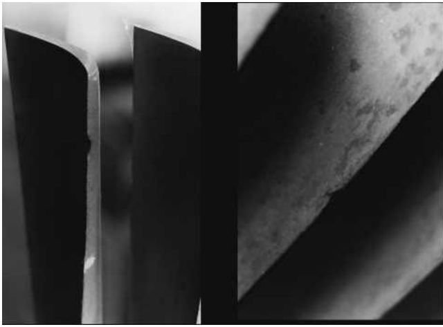
Fig. 12 Droplet eroded LPST blades of 60 MW steam turbine after 15 years of operation
